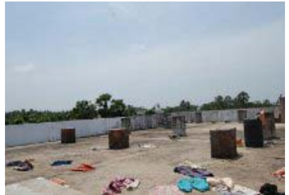
The short base of existing pillars will be what the new pillars will be built on.
